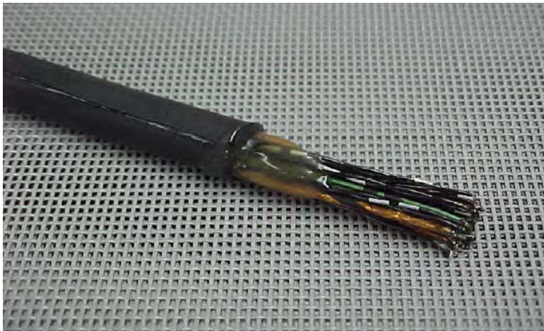
Photo 7: PRT fully shrunk around water blocked end
