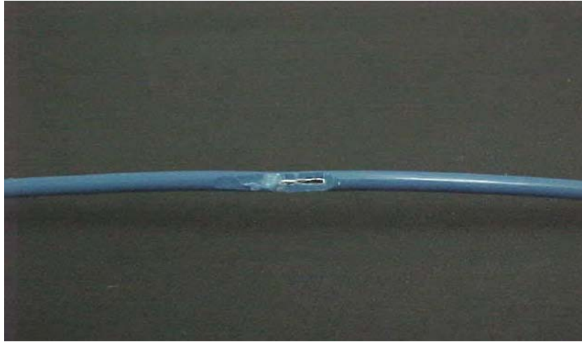
Photo 1: Typical wire or cable insulation damage.
